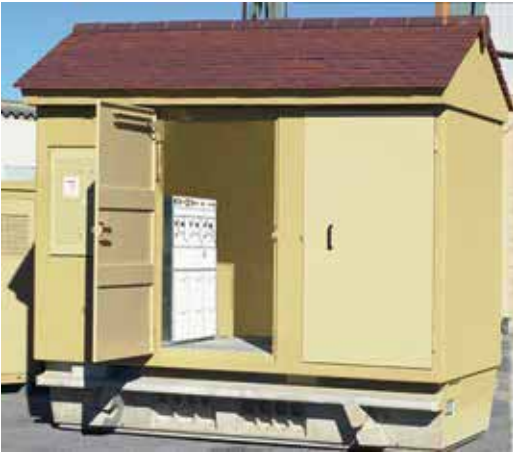
FBX-C in a MV/LV substation – chosen for its compact size
