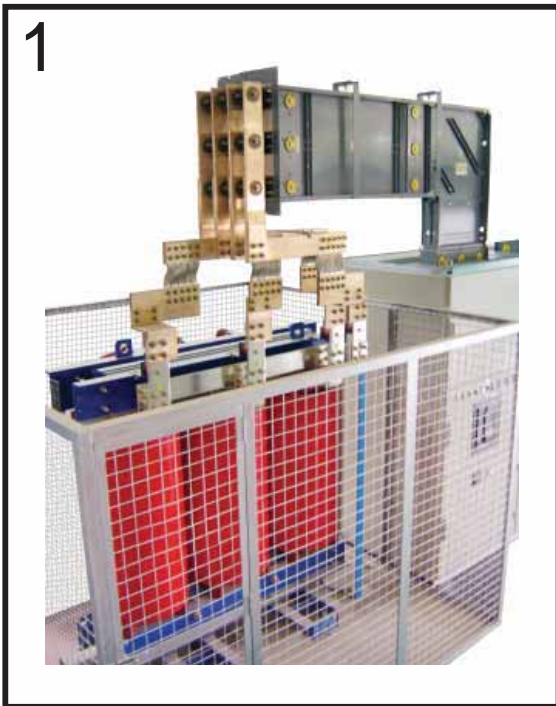
Transformer/ Switchboard connection
