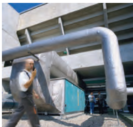
Air handling unit
